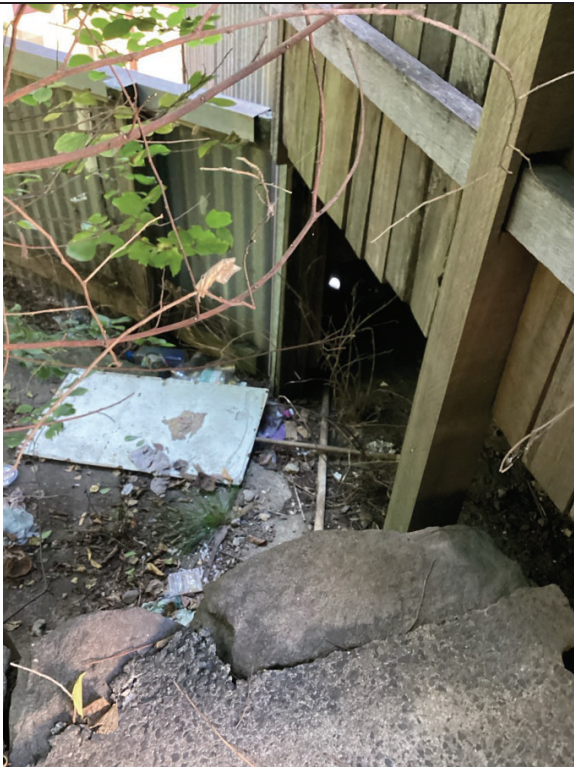
Figure 8 Easement area with void under our client's property
